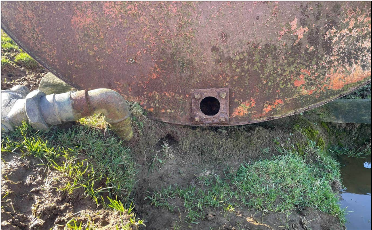
Photograph Appendix B.5: Fittings no longer connected to storage tank, hole at base of tank is rusted.
