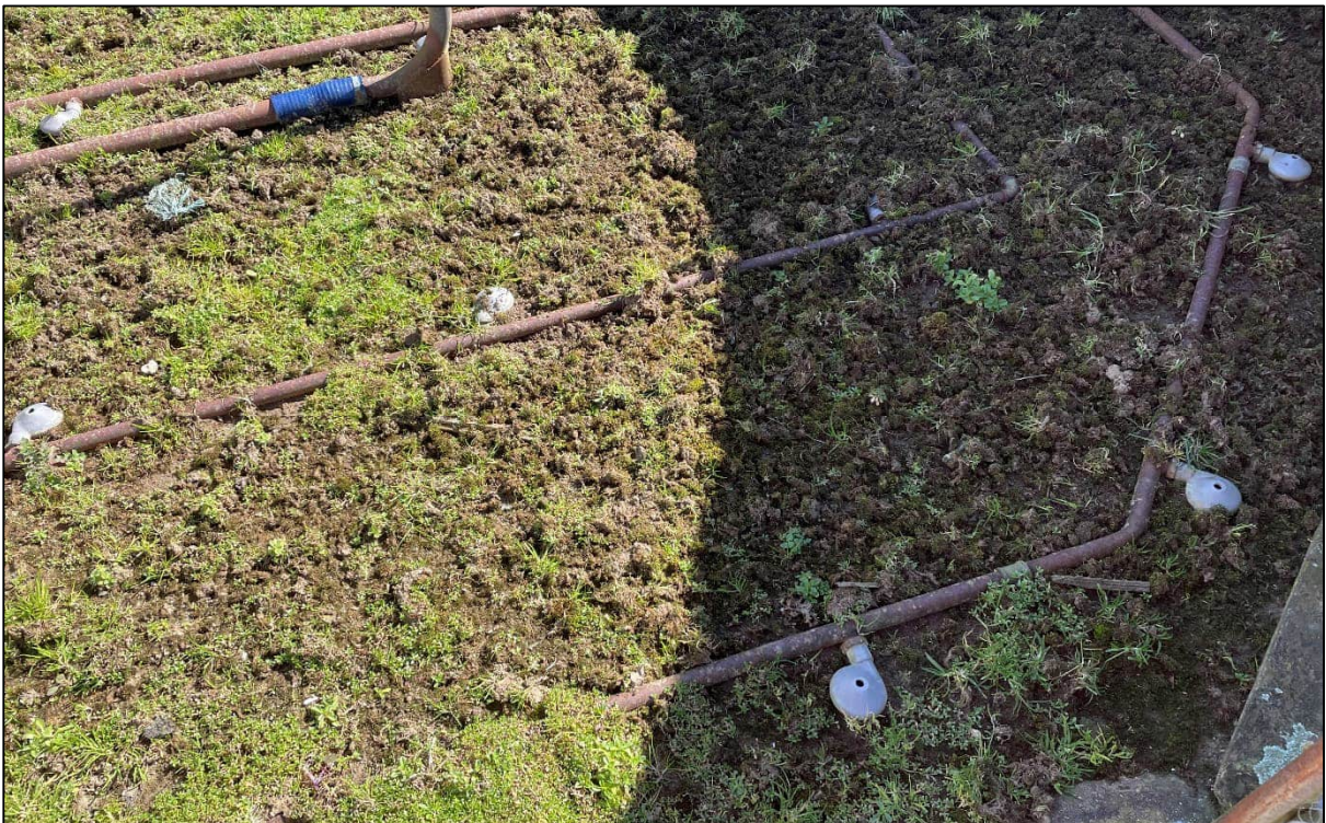
Photograph Appendix B.14: Concrete base of spray sheep dip with pipework, with a layer of sediment and patchy moss and grass cover .
